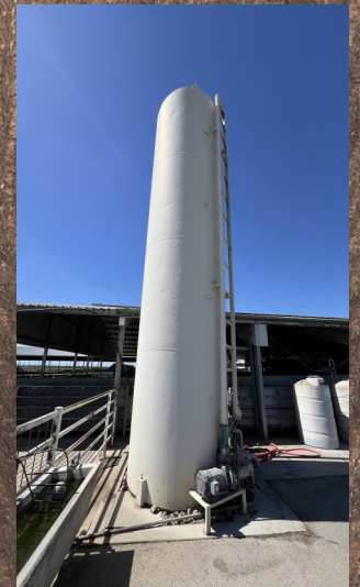
12,000 gallon water storage tank & pump
